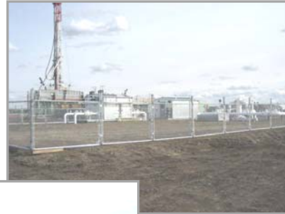
TCPL Meter Station
